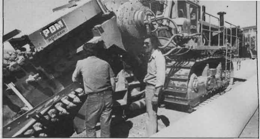
On the Moomba cut the Roc-Saw did the work of six drill and blast crews and cut 2 km a day.
