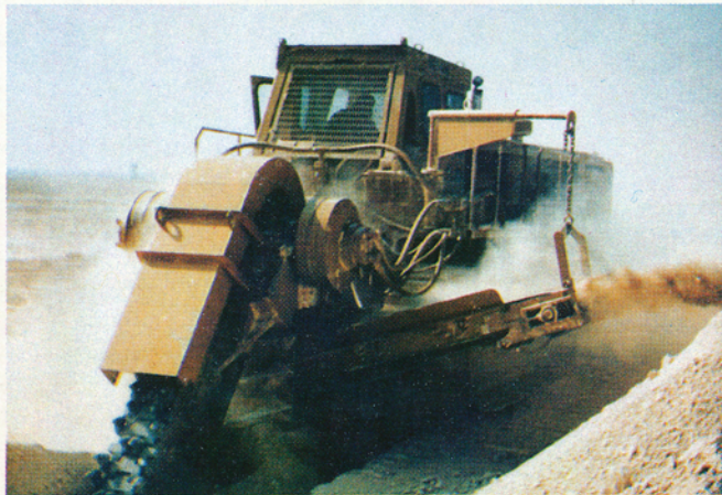
The Roc-Saw cutting through 10,000 psi limestone caprock on the Petromin Pipeline Project in Riyadh, Saudi Arabia. Trenched material was fine enough to backfill into the ditch.
